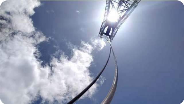
Installation of high-performance Minesform rope on an iconic dragline excavator at the open-cast mines in Queensland, Australia.
