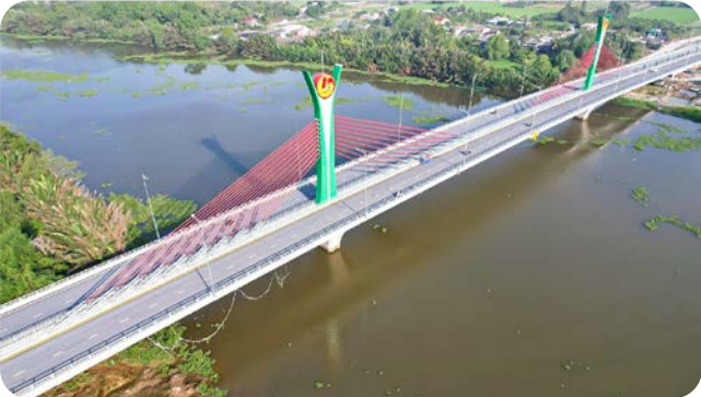
Installation of high-quality galvanised LRPC strands in Vam Co Tay Bridge in Vietnam.
