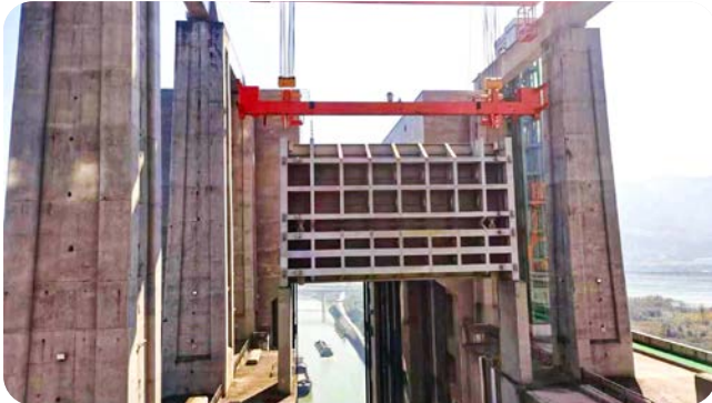
Installation of Powerform crane ropes on the Three Gorges Dam in China, which is the largest power station in the world by installed capacity.
